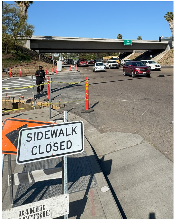
Sidewalk closures and improper crossings during construction near SR-125 off-ramps
